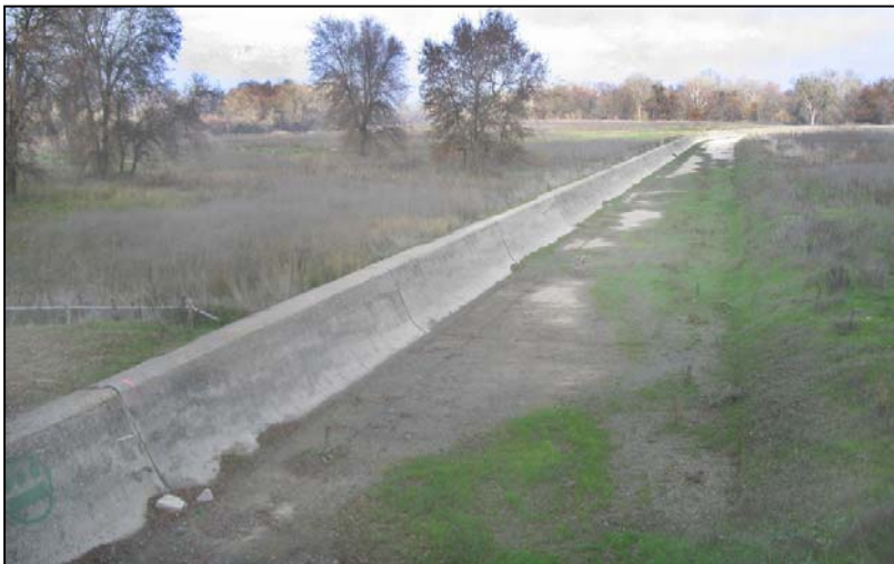
Figure 47. Flow (left to right) over Fremont Weir (looking east) during the 2006 flood.
